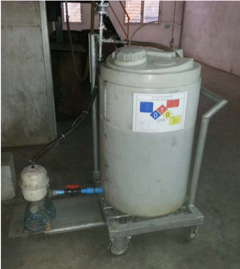
Dosing pump and tank
